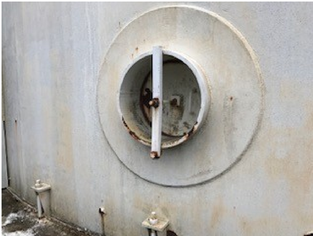
Existing manway access hatch to be removed and replaced with new 30" bolt down flanged hatch.
