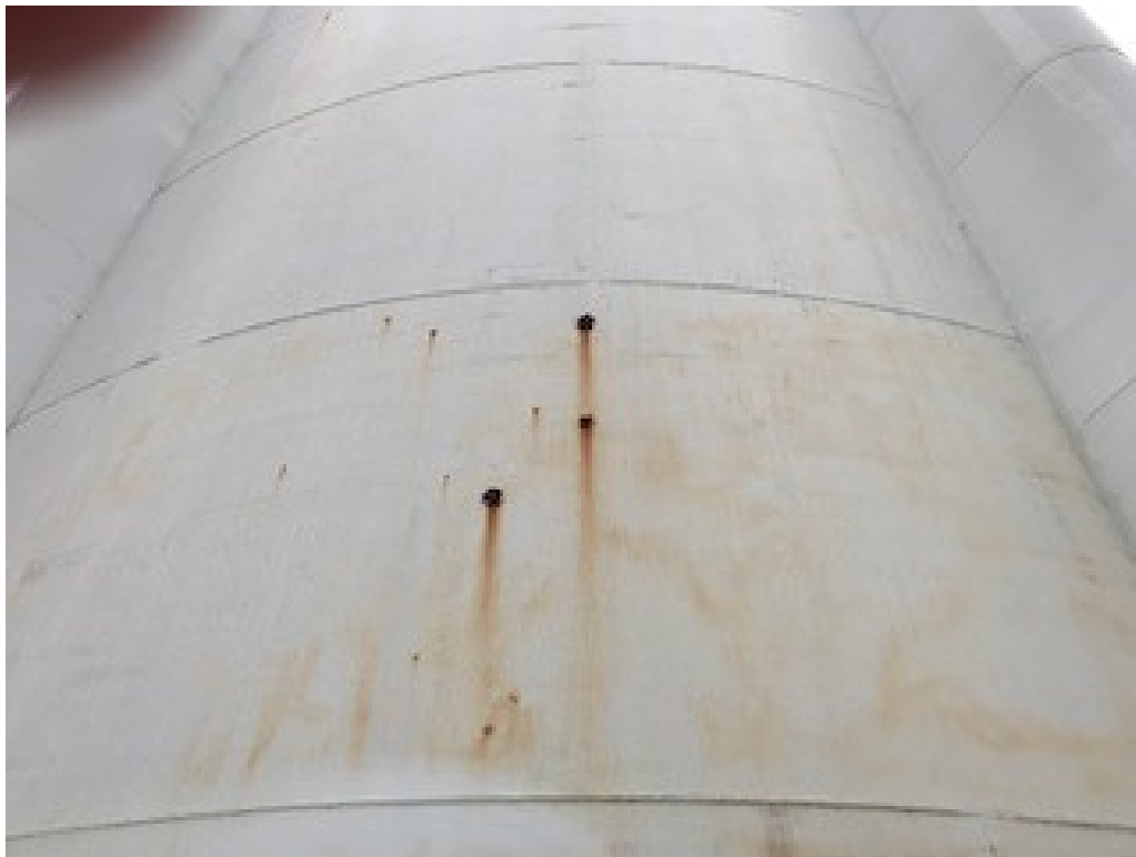
Delamination of exterior coating system.
