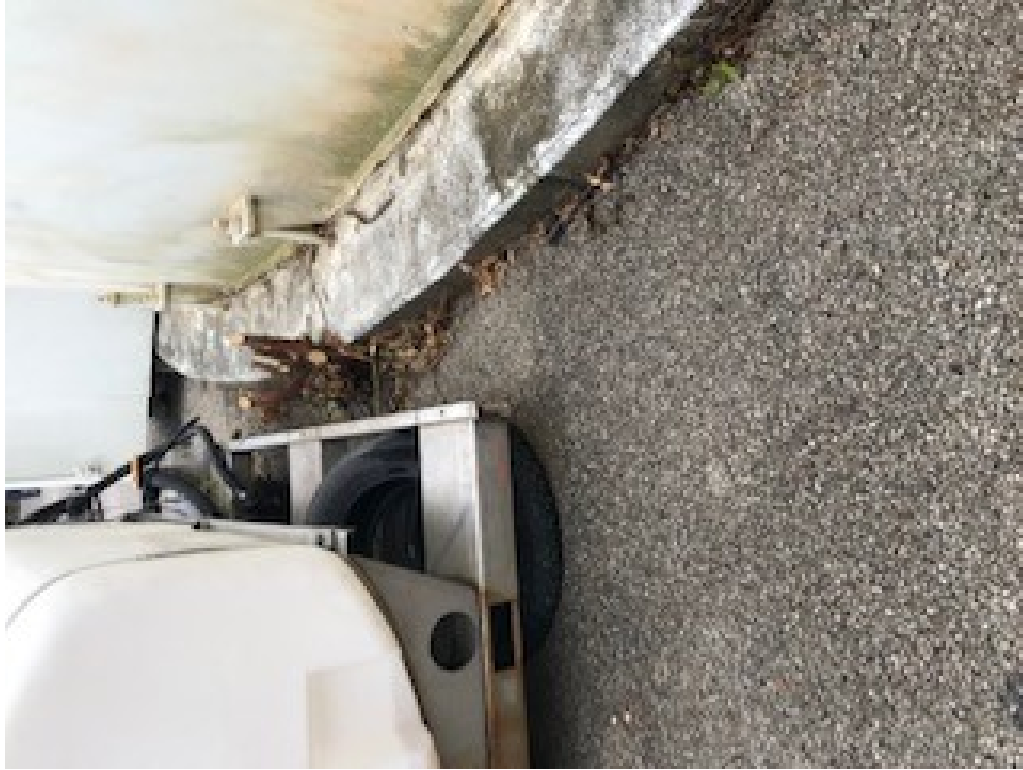
Foundation ring wall of standpipe and anchor bolts and chairs to be blasted and repainted.
