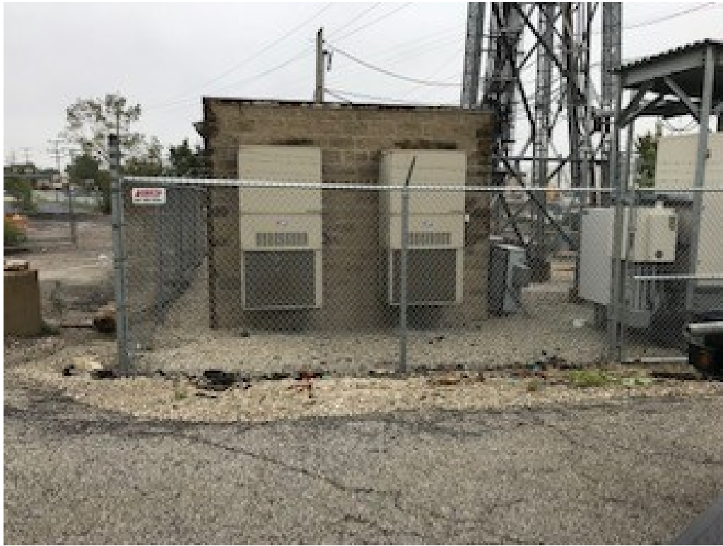
Communications equipment building located at southwest corner of site. Contractor to keep area clear.
