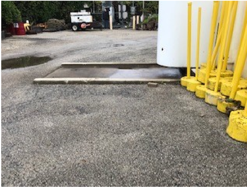
Splash block to be maintained to overflow piping.
