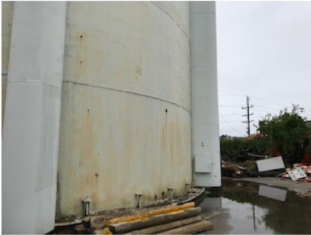
North side of standpipe showing delamination of exterior coating surface.
